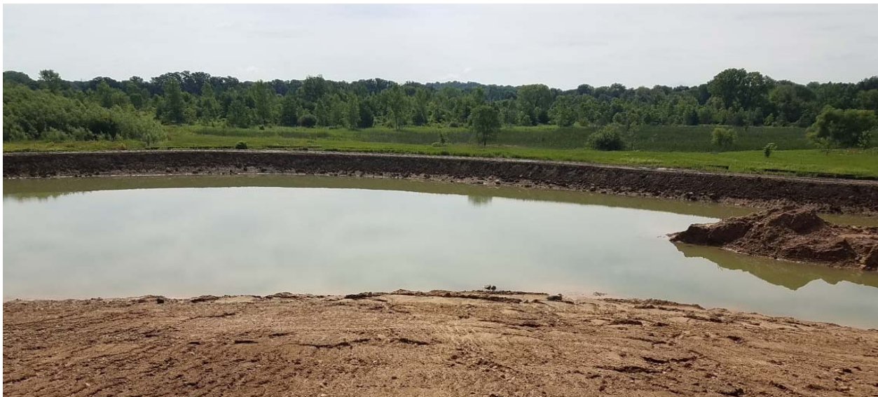
Figure 2: The photo above was taken on June 30 th showing the excavation in the area of bioinfiltration. Note the berm on the far side of the water. The berm will be trimmed back to match the slope in a later phase of the project.
