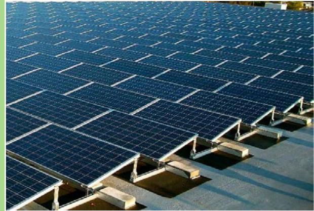
Example of a rooftop installation
