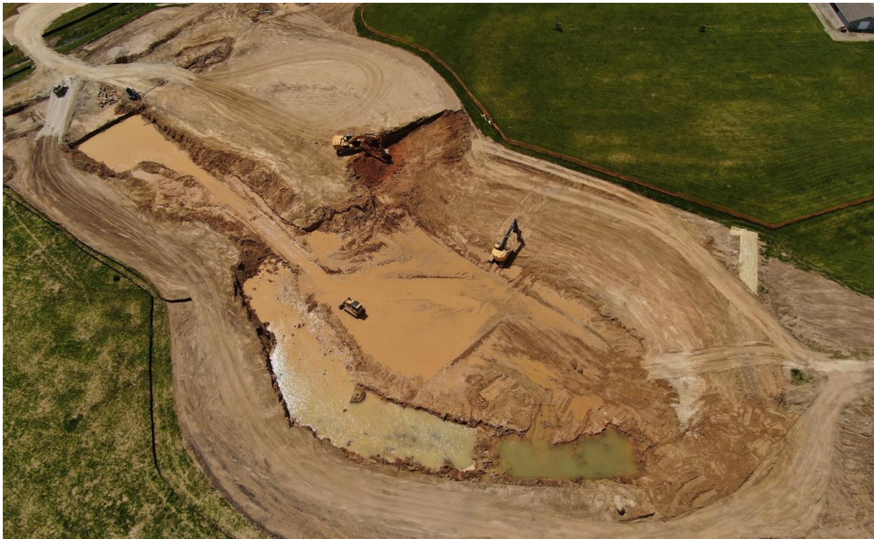
Figure 2: Drone photo showing the extent of the excavation as of May 14th, 2021. The basin excavation has merged with the temporary sedimentation basin. Photo by Jon Bublitz.
