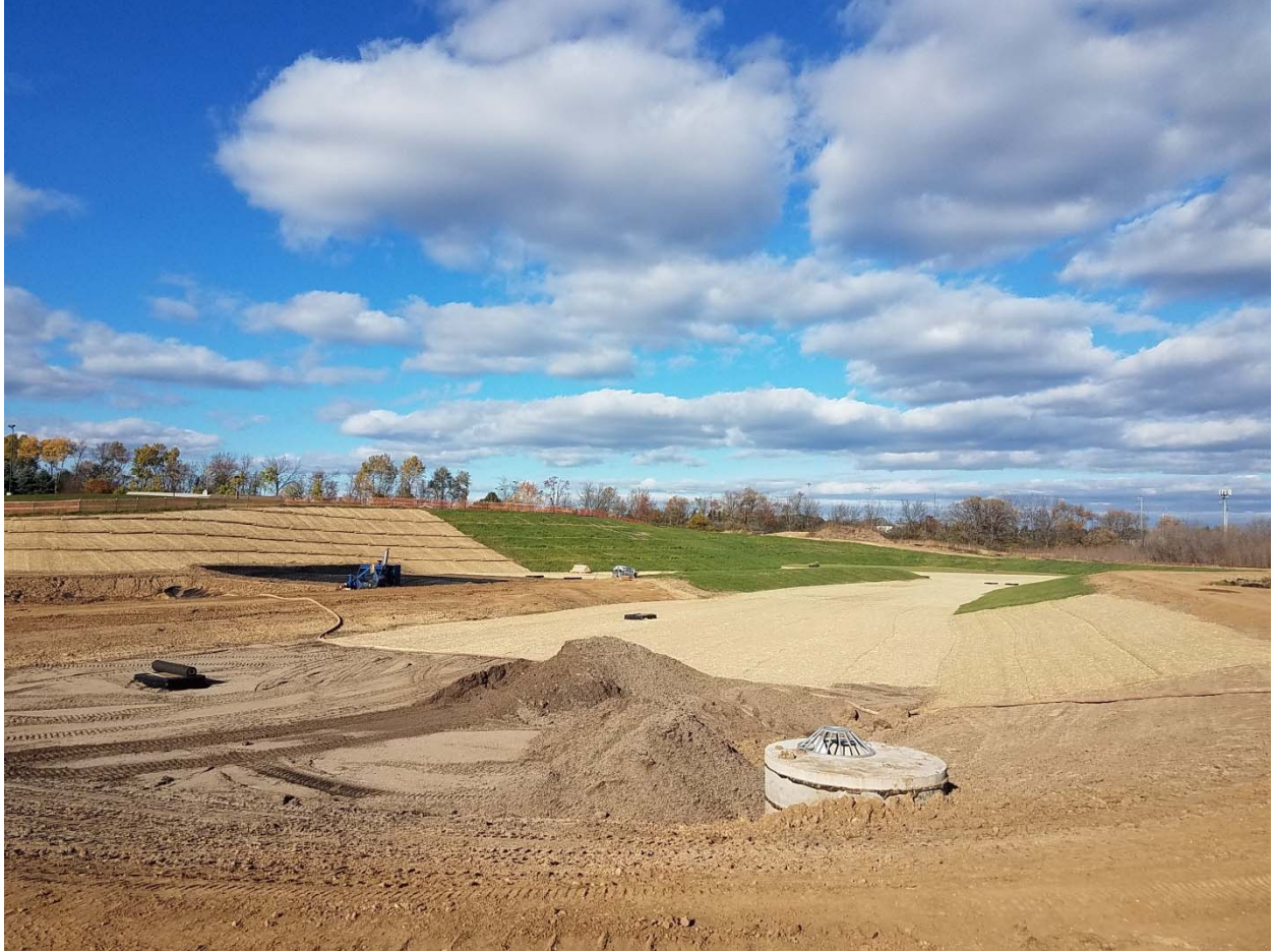
Figure 2: Engineered soil in the biofiltration basin has been seeded and erosion mat placed over the top. Photo taken 11/3/21.
